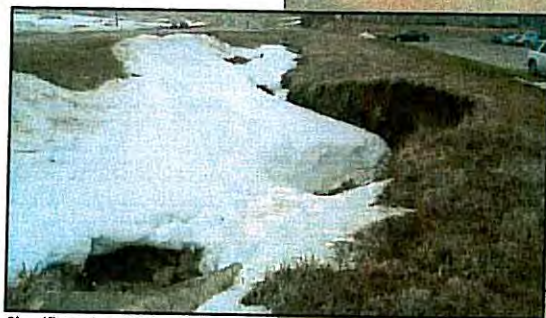
Significant cutting and scouring at southern outfall into swale looking north.
